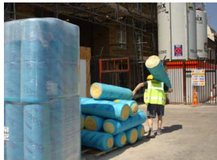
Materials which could have been unloaded directly into site storage areas are instead carried by hand from temporary storage in the street
