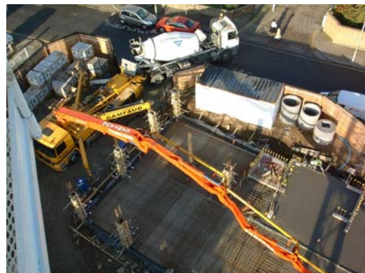
Aerial view of Ready Mixed concrete being transferred from the delivery vehicle and pumped into positioned
