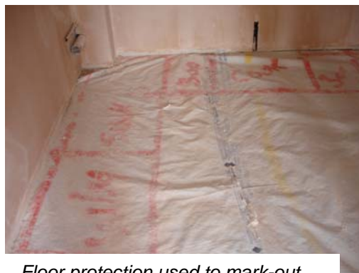
Floor protection used to mark-out positions of kitchen units, radiator positions and pipe runs
