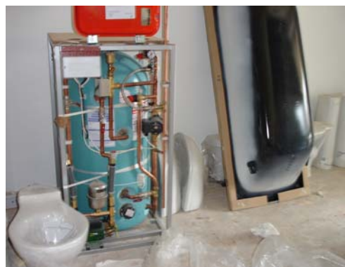
Sanitary ware and a boiler positioned ready for skilled trades to commence fitting
