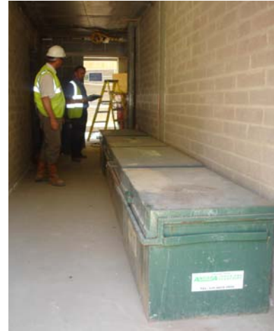
Trade contractor lock-up boxes giving easy access to tools or and small components
