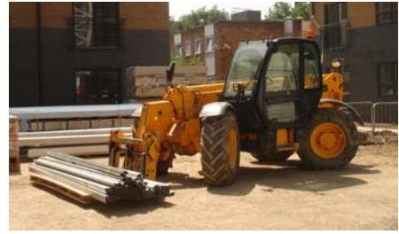
The forklift is able to position materials directly onto loading bays at high level
