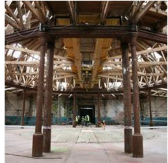
Derby Roundhouse for Derby College, Constructing Excellence East Midlands Regional Project of the Year 2009, and National Runner-Up
