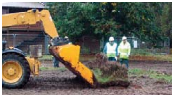
Translocation of an area of heather which was found to support 10% of the UK population of Nightjar and Woodlark
