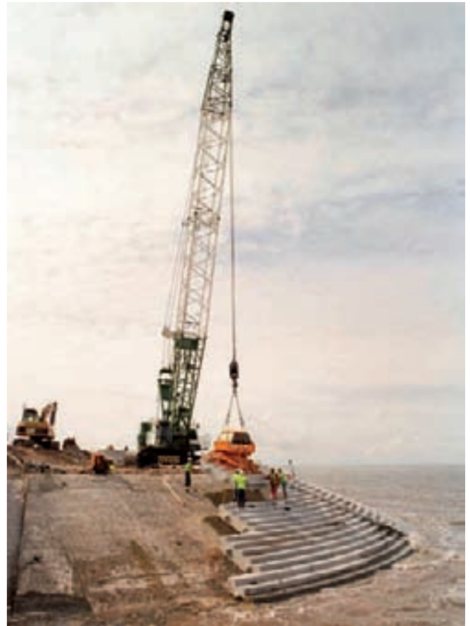
New Coastal Defence Revetment Works: Use of 135T Crawler Crane and Specialist Vacuum Lifting Unit to install 15.5T Precast Stepped Revetment Units during limited tidal working period
