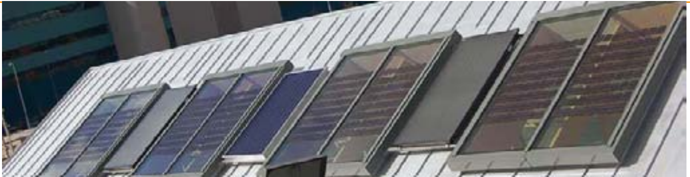
South facing roof featuring both solar thermal and photovoltaic installations
