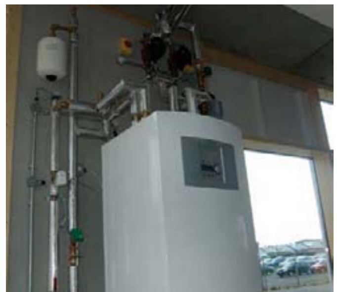
Worcester Ground source heatpump
