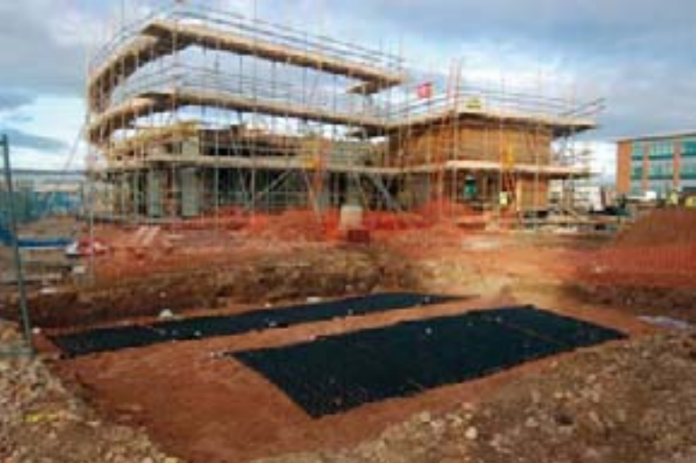
Eastern elevation showing ground source heatpump compact collectors
