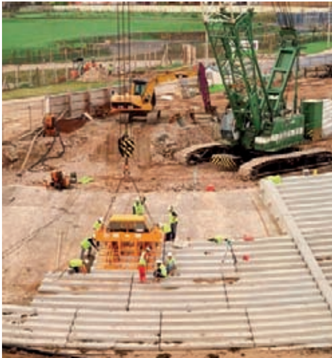
New Coastal Defence Revetment Works: Placement and Bedding of curved Precast Stepped Revetment Units to prepared Revetment Substructure
